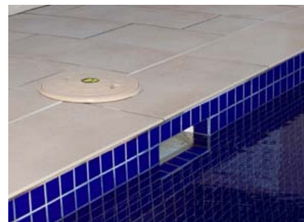
Figure 9. The skimmer is the port that draws water from the pool and into the filtration system.
